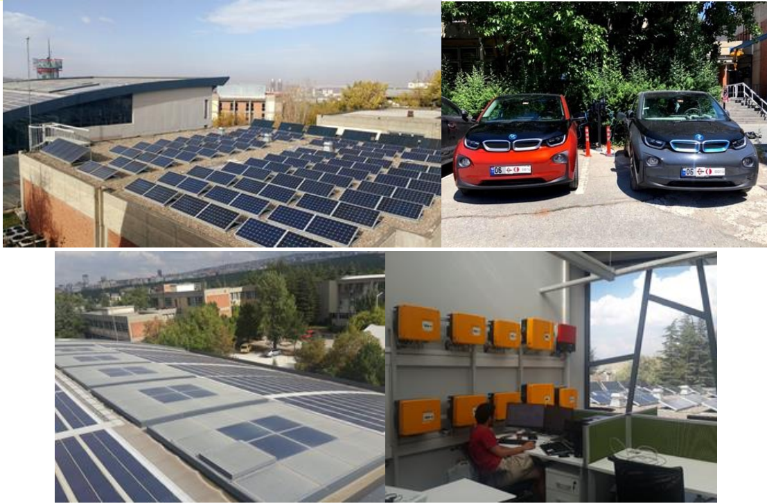
Fig -1: 25 kW rooftop grid connected PV systems and 2 electric car charging stations.
